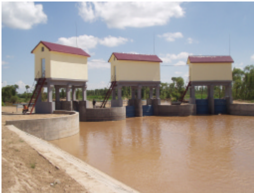
Photo 2 Water gate on Yongji Main Canal from which Xile Secondary Canal takes off
