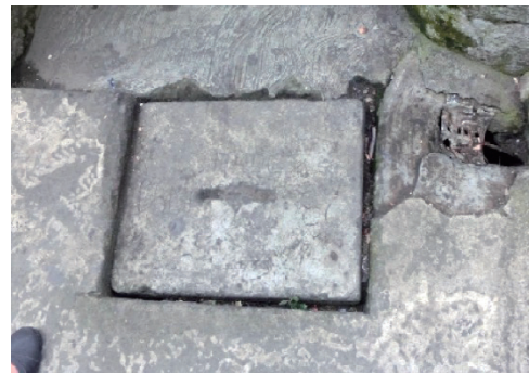
Figure 9. Underground sewer ( gorong-gorong ).
