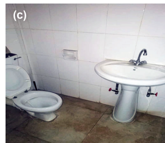
(c) An improved toilet in Zambia with a hand washing station installed in the toilet room.
